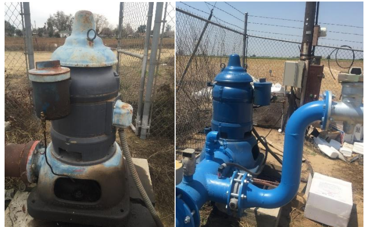
Figure 2. Turbine pump on a small-scale Southeast Asian farm, before and after improvements to increase energy efficiency funded by SWEET
